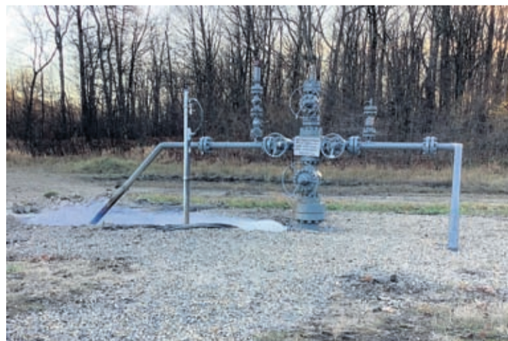
This Nov. 7, 2022, photo, released by the Pennsylvania Department of Environmental Protection shows a methane leak at a well owned by Equitrans Midstream at their Rager Mountain storage facility near Jackson Township, Pa.
